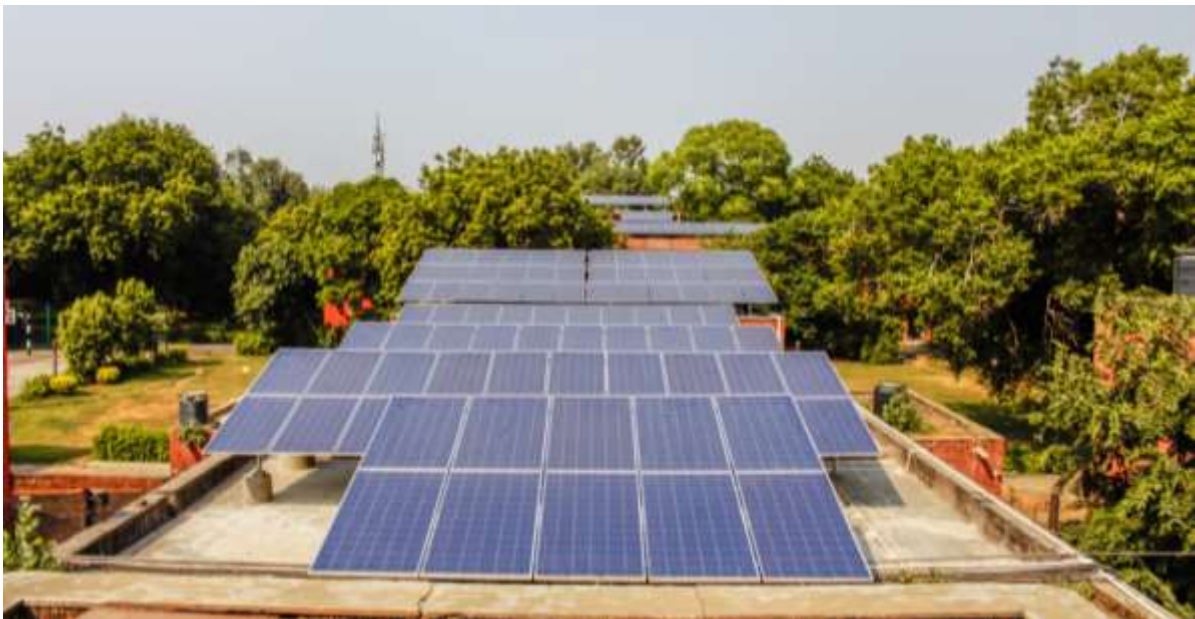
218 kWp Solar Power Plant at Lady Irwin College, inaugurated by Hon'ble Chief Minister, Govt. of NCT of Delhi on 14 th October'2020
